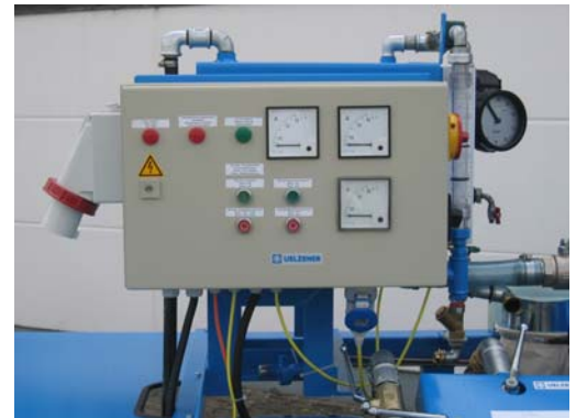
Electric control box
