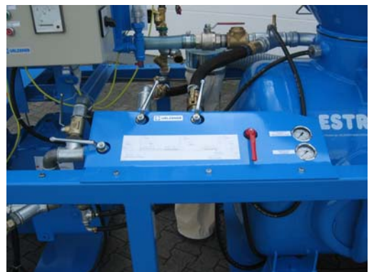
Compressed air control armatures
