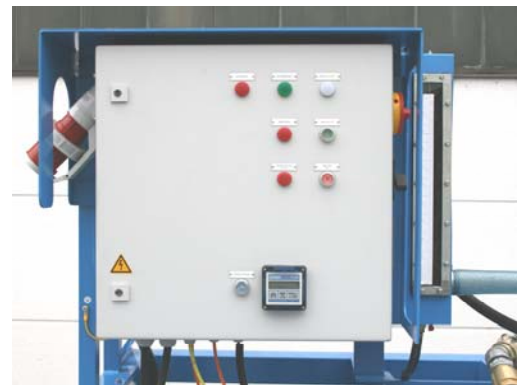
Electric control box
